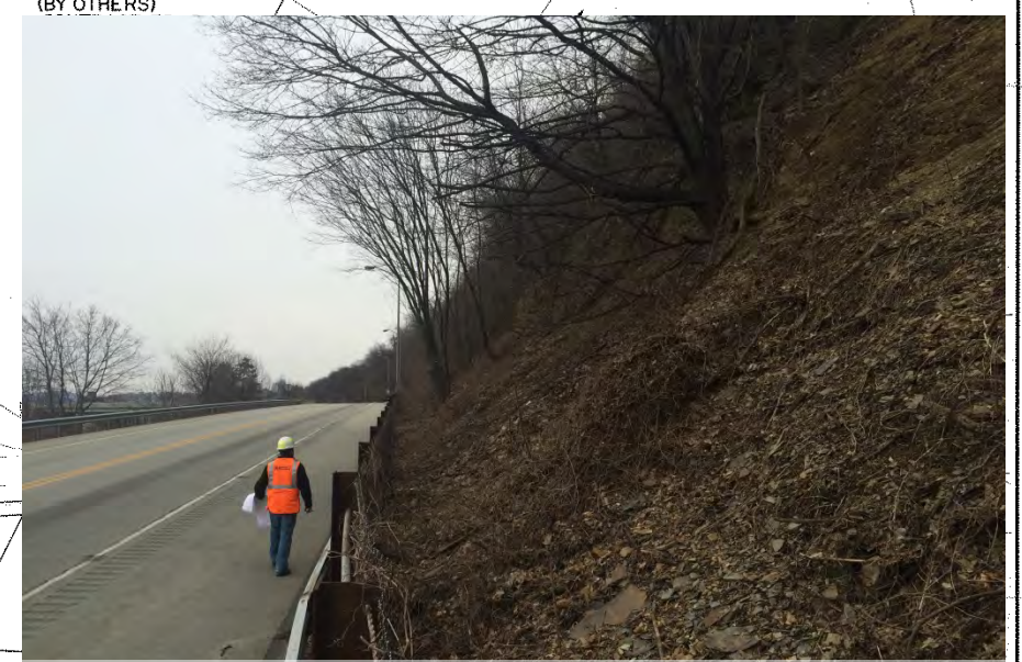
TALUS BUILD UP BEHIND ROCKFALL BARRIER. CATCHMENT AREA IS COMPLETELY FILLED AND BARRIER IS SERVING AS RETAINING WALL
